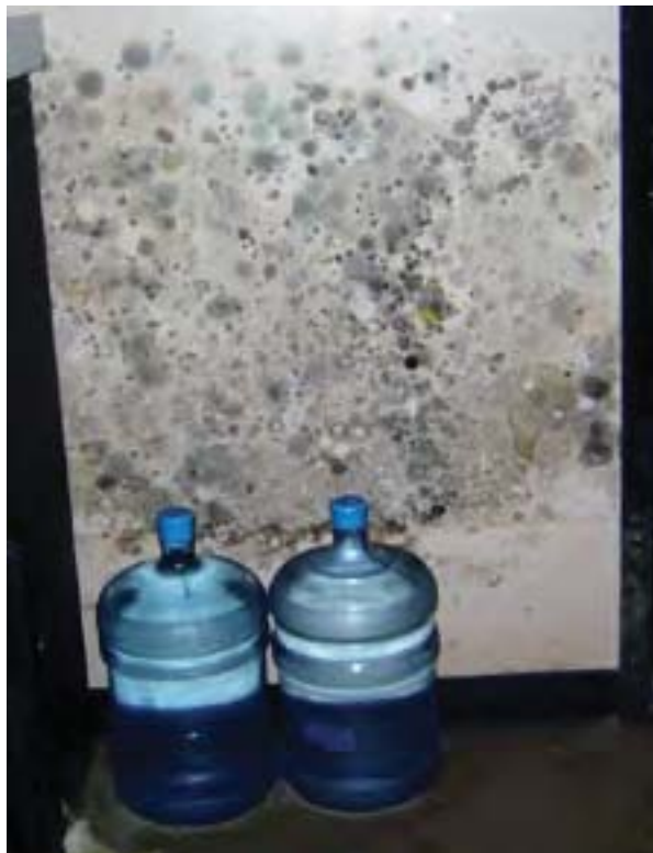
Mold growth on wall board.
