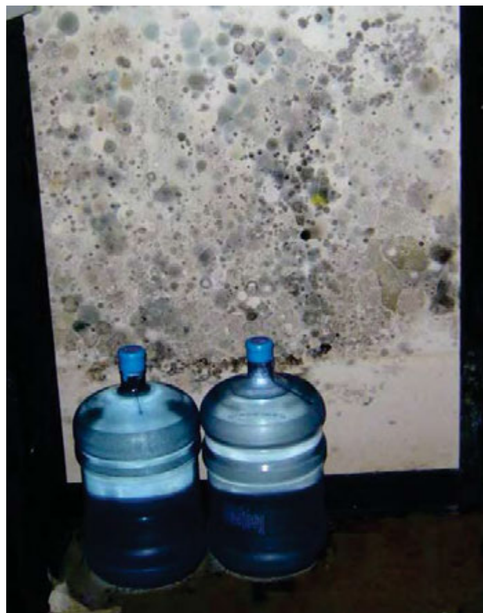
Mold growth on wall board.
